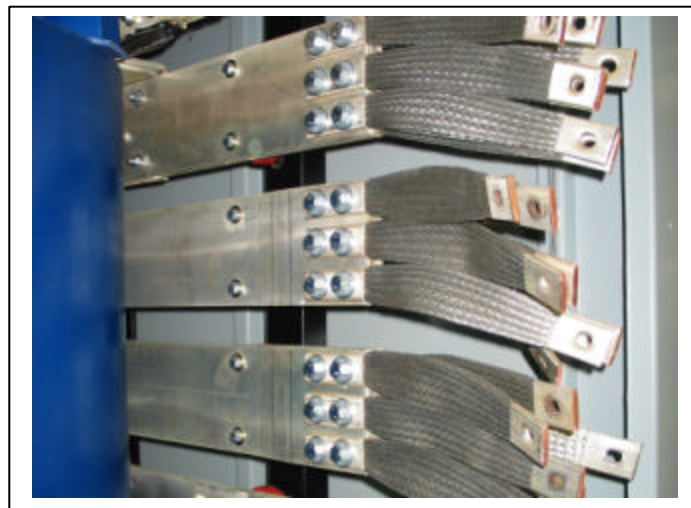
Typical 600V class transformer - switchgear connection
